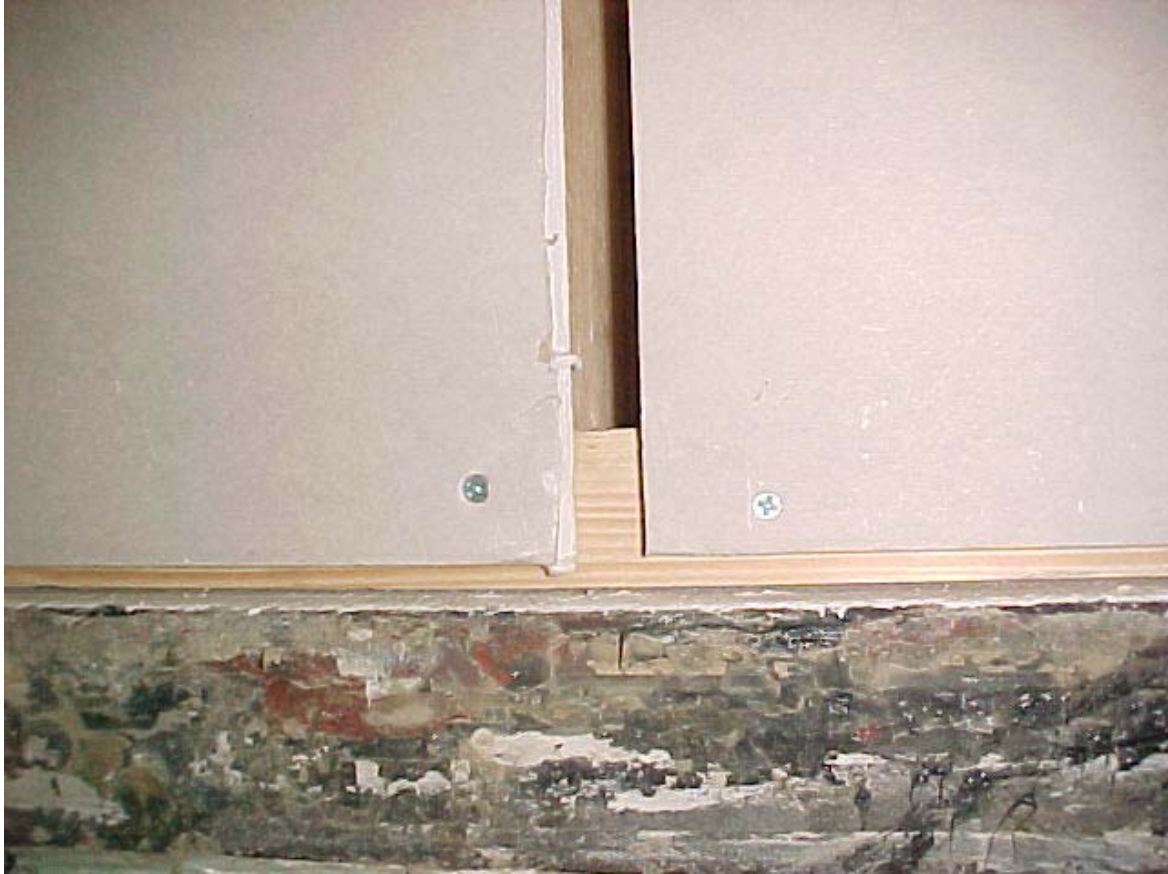
Photograph 2: Unsealed Partition Close-Up
