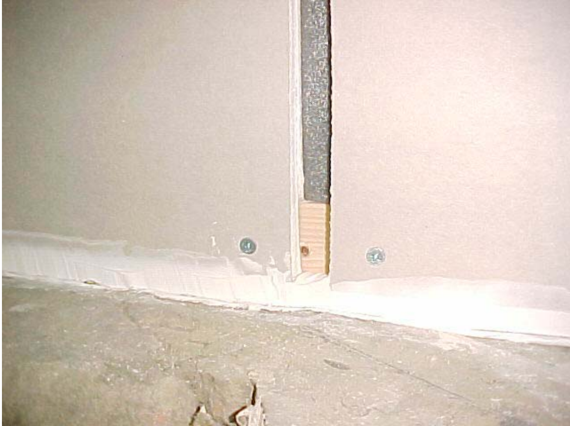
Photograph 3: Partially Unsealed Partition Close-Up
